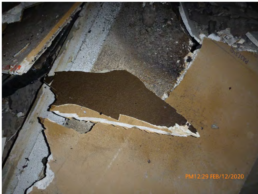
Photograph 27: February 12, 2020, at approximately 12:29 PM - View of textured drywall in a debris pile inside the north room of Unit 3. The material was sampled and later determined to contain 2% Chrysotile Asbestos by the point count method using polarized light microscopy. The material was in a dry condition with no evidence of moisture.
