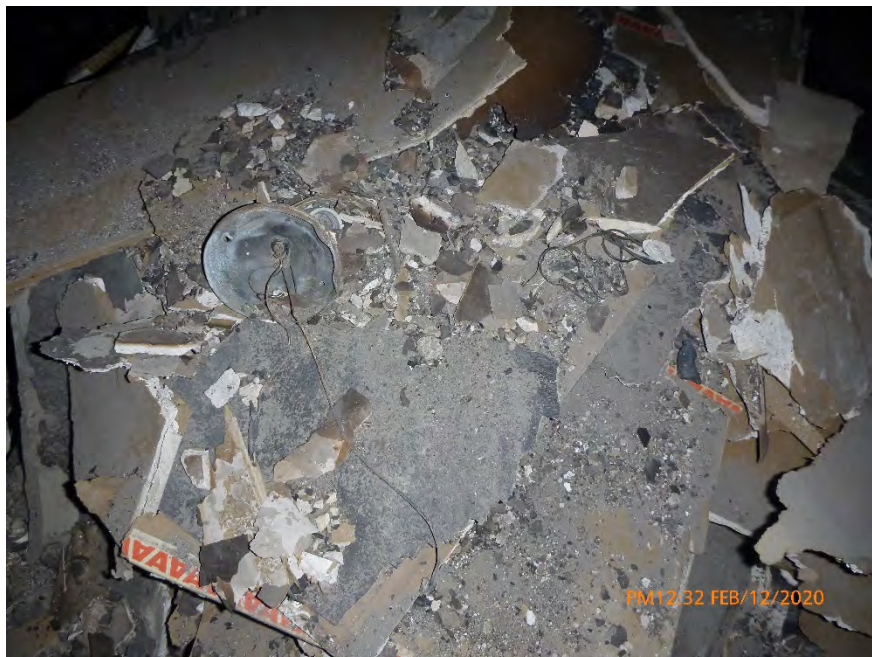
Photograph 29: February 12, 2020, at approximately 12:32 PM - View of textured drywall in a debris pile inside the north room of Unit 3. The material was sampled and later determined to contain 2% Chrysotile Asbestos by the point count method using polarized light microscopy. The material was in a dry condition with no evidence of moisture.
