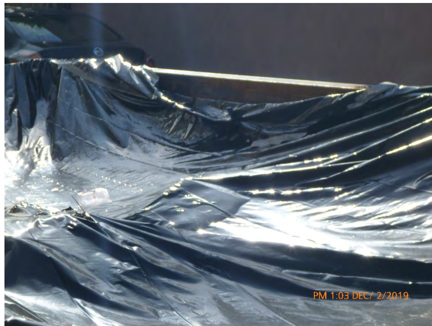
Photograph 27: December 2, 2019, at approximately 1:03 PM - View of the 16 cubic yard dumpster which contains ACWM. The dumpster is no longer sealed.
