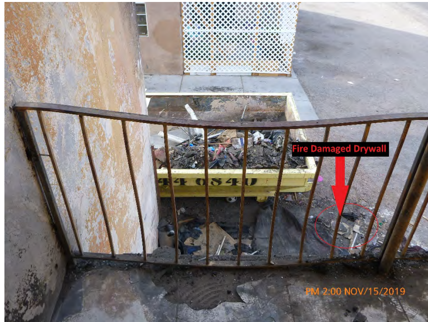
Photograph 13: November 15, 2019, at approximately 2:00 PM - View of the balcony of the north room of Unit #3 overlooking the 16 cubic yard dumpster. Note the accumulation of fire damaged debris along the bottom edge of the guard rail which suggests the fire damaged debris was swept over the edge. Also note the presence of fire damaged drywall on the pavement adjacent to the dumpster.
