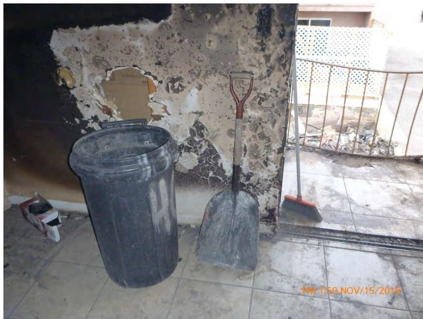
Photograph 12: November 15, 2019, at approximately 1:59 PM – View of a waste bin, a wide mouth shovel, and a broom in the north room of Unit #3. Note the absence of fire damaged debris in the photograph. Shovels like the one depicted in the photograph are typically used for the removal of materials such as soil, ash, ACT debris, etc...
