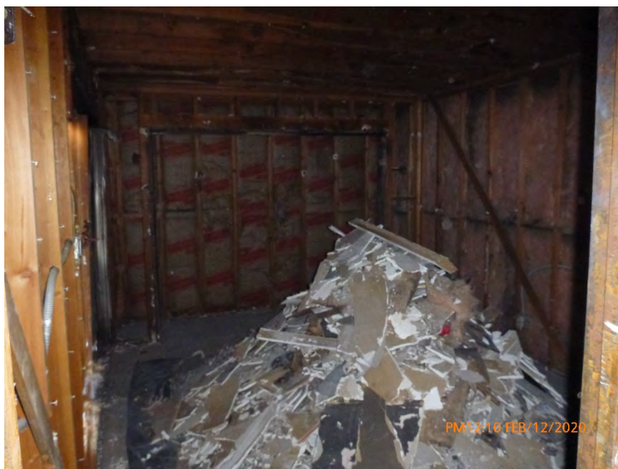
Photograph 22: February 12, 2020, at approximately 12:10 PM - View of Asbestos-Containing Waste Material ( ACWM ) inside of the north room of Unit 3. The ACWM was in a dry condition with no evidence of moisture. Textured drywall, including acoustic ceiling texture, had been removed from all of the walls and ceilings. The texture on the walls and ceilings were Regulated Asbestos-Containing Materials.
