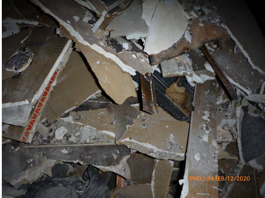
Photograph 33: February 12, 2020, at approximately 12:20 PM - View of textured drywall in a debris pile inside the north room of Unit 3. The material was sampled and later determined to contain 2% Chrysotile Asbestos by the point count method using polarized light microscopy. The material was in a dry condition with no evidence of moisture.
