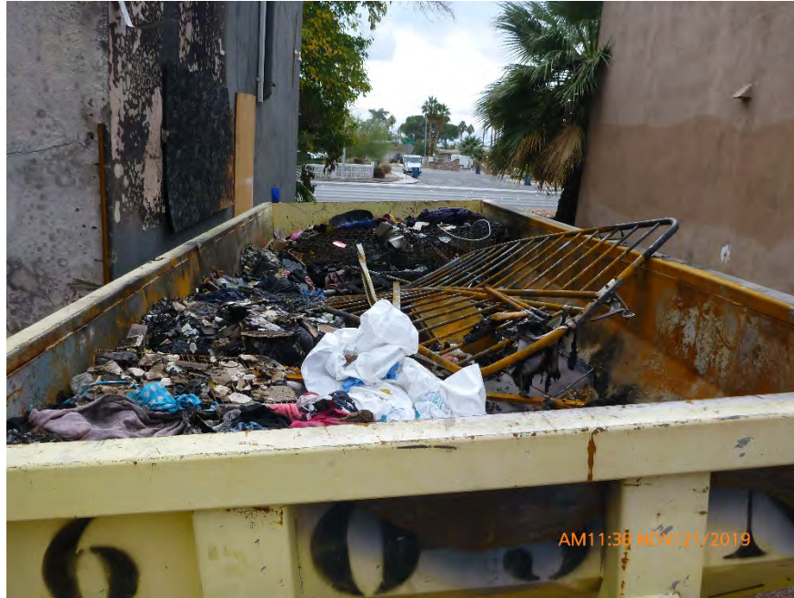
Photograph 24: November 21, 2019, at approximately 11:30 AM - View of the 16 cubic yard dumpster which contains ACWM. The dumpster remains uncovered and is not posted with asbestos warning signs.
