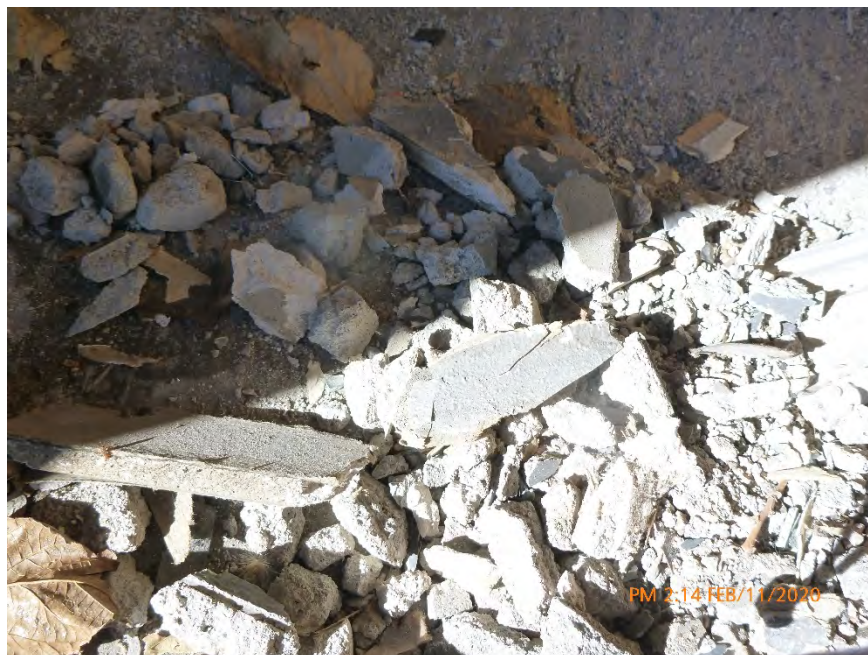
Photograph 19: February 11, 2020, at approximately 2:14 PM – View of textured drywall debris on the south/living room patio of Unit 1. The material was sampled and later determined to contain 2% Chrysotile Asbestos by polarized light microscopy. The material was in a dry condition with no evidence of moisture.
