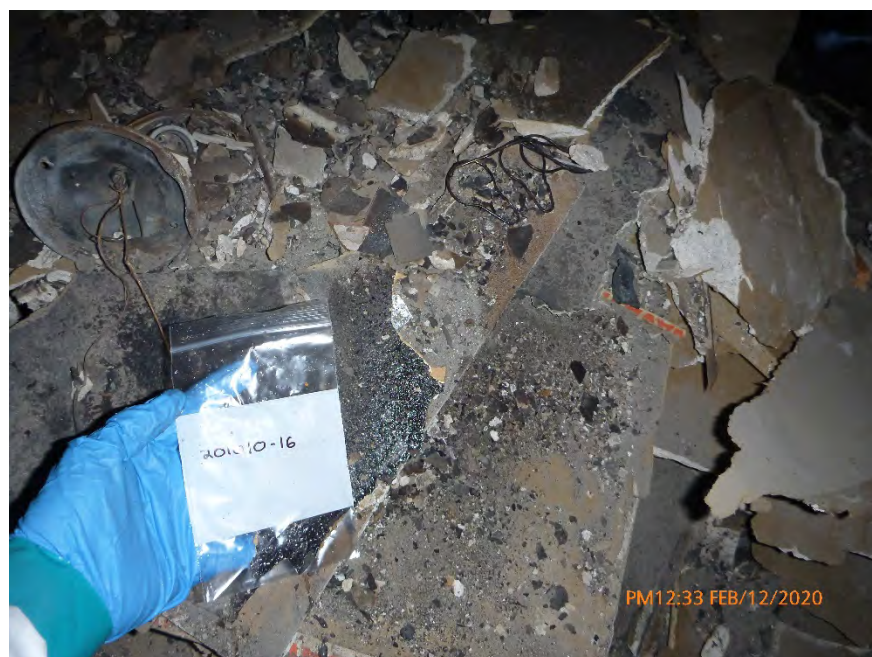
Photograph 30: February 12, 2020, at approximately 12:33 PM - View of Sample #201010-16 obtained from the material depicted in Photograph #29.
