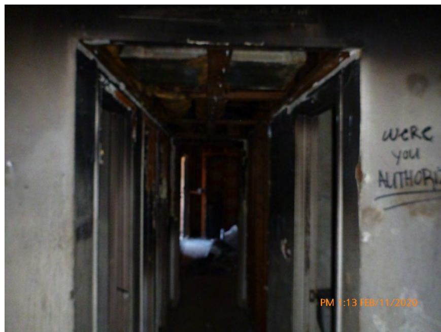
Photograph 4: February 11, 2020, at approximately 1:13 PM - View of a hallway in Unit 1 where textured drywall, including acoustic ceiling texture, had been removed from the west wall and ceiling. The texture on the walls and ceilings were Regulated Asbestos-Containing Materials.
