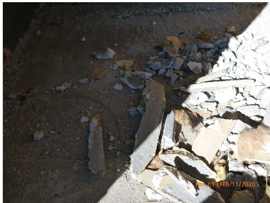
Photograph 17: February 11, 2020, at approximately 2:13 PM – View of textured drywall debris on the south/living room patio of Unit 1. The material was sampled and later determined to contain 2% Chrysotile Asbestos by polarized light microscopy. The material was in a dry condition with no evidence of moisture.
