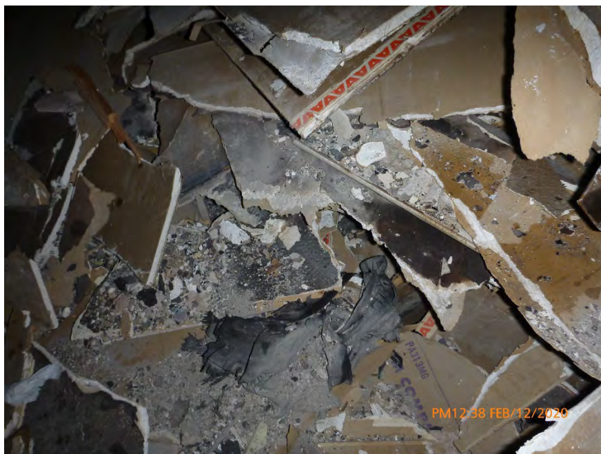
Photograph 35: February 12, 2020, at approximately 12:38 PM - View of textured drywall in a debris pile inside the north room of Unit 3. The material was sampled and later determined to contain 3% Chrysotile Asbestos by the point count method using polarized light microscopy. The material was in a dry condition with no evidence of moisture.
