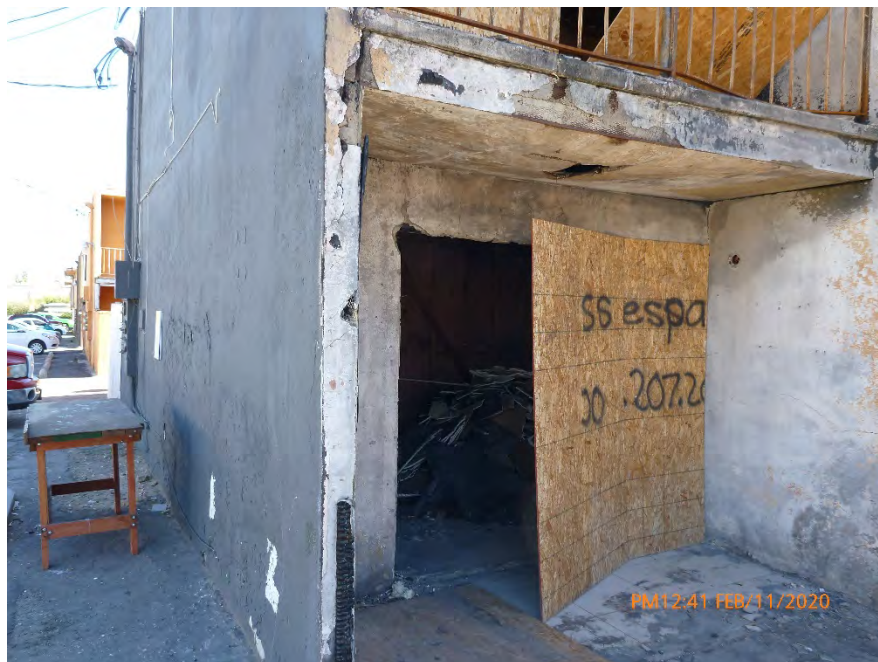
Photograph 1: February 11, 2020, at approximately 12:41 PM - View of the patio entrance to Unit 1. Plywood boards used to secure the entrance have been removed and no asbestos warning signs are posted. The Asbestos-Containing Waste Material inside is exposed to the outside air and is accessible to the public.
