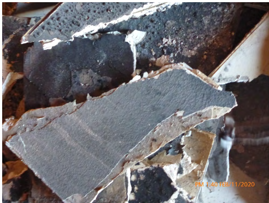
Photograph 13: February 11, 2020, at approximately 1:40 PM - View of textured drywall in a debris pile inside the north room of Unit 1. The material was sampled and later determined to contain 4% Chrysotile Asbestos by the point count method using polarized light microscopy. The material was in a dry condition with no evidence of moisture.
