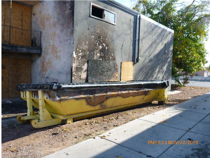
Photograph 26: November 22, 2019, at approximately 12:23 PM - View of the 16 cubic yard dumpster which contains ACWM. The dumpster is sealed but asbestos warning signs are not posted.
