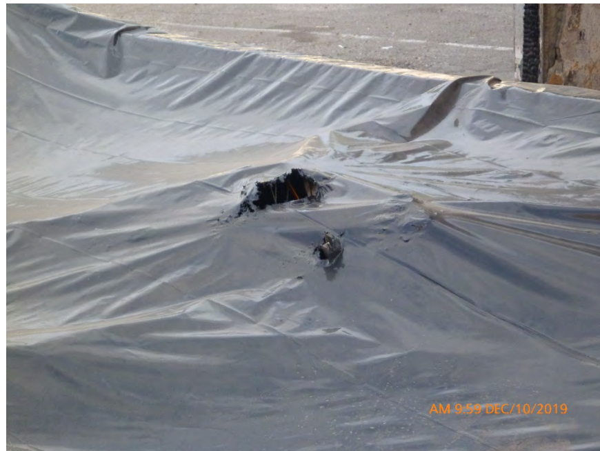
Photograph 29: December 10, 2019, at approximately 9:59 AM - View of the 16 cubic yard dumpster which contains ACWM. The dumpster is no longer sealed.
