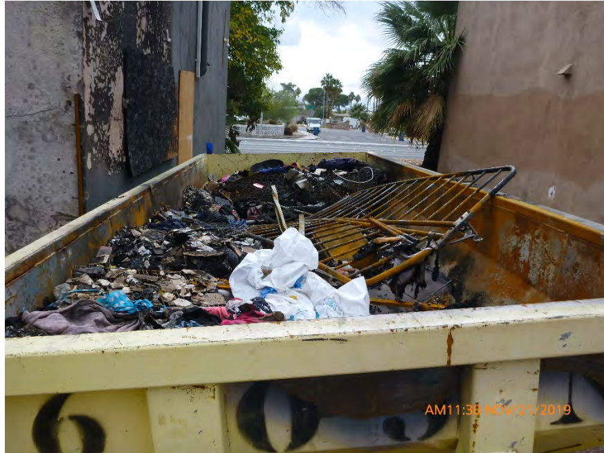
Photograph 24: November 21, 2019, at approximately 11:30 AM - View of the 16 cubic yard dumpster which contains ACWM. The dumpster remains uncovered and is not posted with asbestos warning signs.
