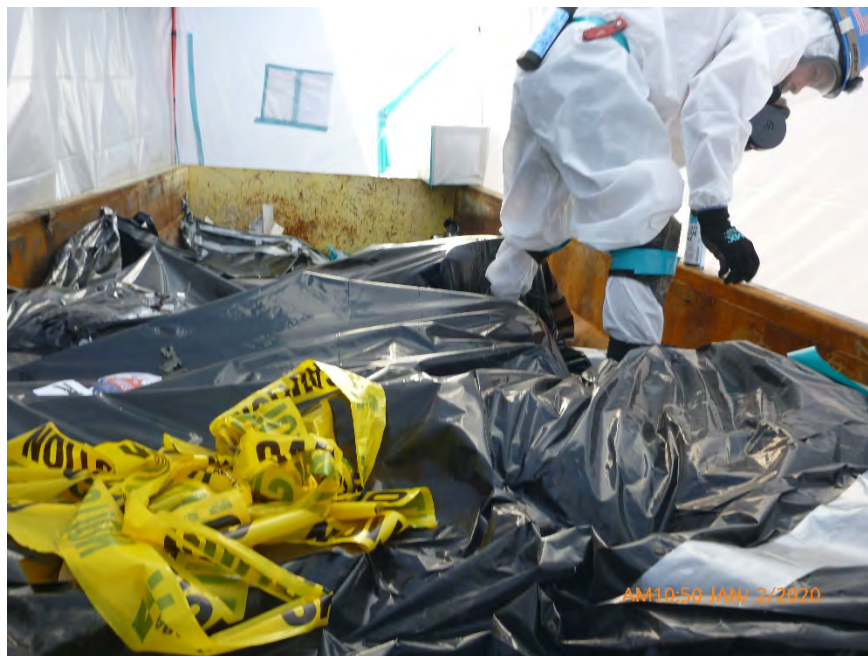
Photograph 31: January 2, 2020, at approximately 10:50 AM - View of an asbestos worker setting up containment in preparation for the abatement of the 16 cubic yard dumpster which contained ACWM.
