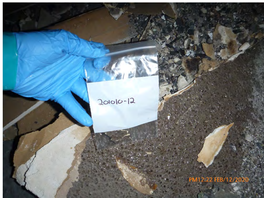
Photograph 26: February 12, 2020, at approximately 12:22 PM - View of Sample #201010-12 obtained from the material depicted in Photograph #25.
