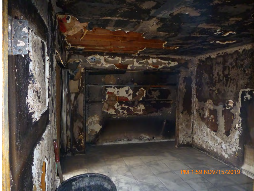
Photograph 11: November 15, 2019, at approximately 1:59 PM – View of the north room (master bedroom) of Unit #3. Nearly all of the ACT is missing and there are several holes in the ceiling. Despite the missing materials, the floor of the north room in Unit #3 contained almost no debris.
