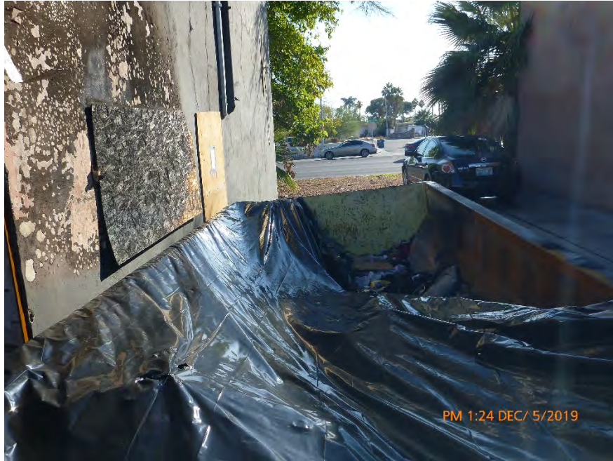
Photograph 28: December 5, 2019, at approximately 1:24 PM - View of the 16 cubic yard dumpster which contains ACWM. The dumpster is no longer sealed and debris has been removed (See Photograph #24 regarding the amount of material that was previously in the dumpster).
