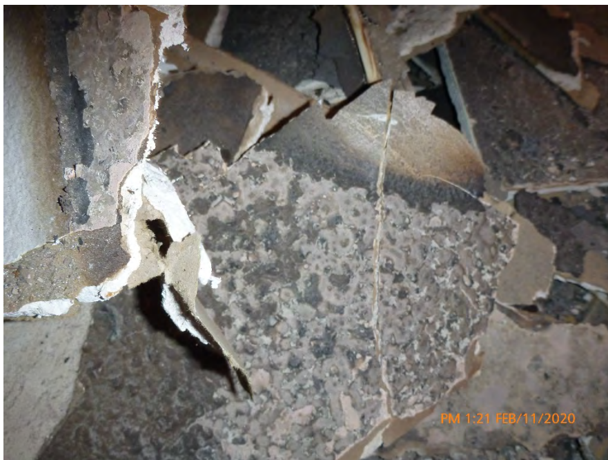
Photograph 7: February 11, 2020, at approximately 1:18 PM - View of textured drywall in a debris pile inside the north room of Unit 1. The material was sampled and later determined to contain 2% Chrysotile Asbestos by the point count method using polarized light microscopy. The material was in a dry condition with no evidence of moisture.
