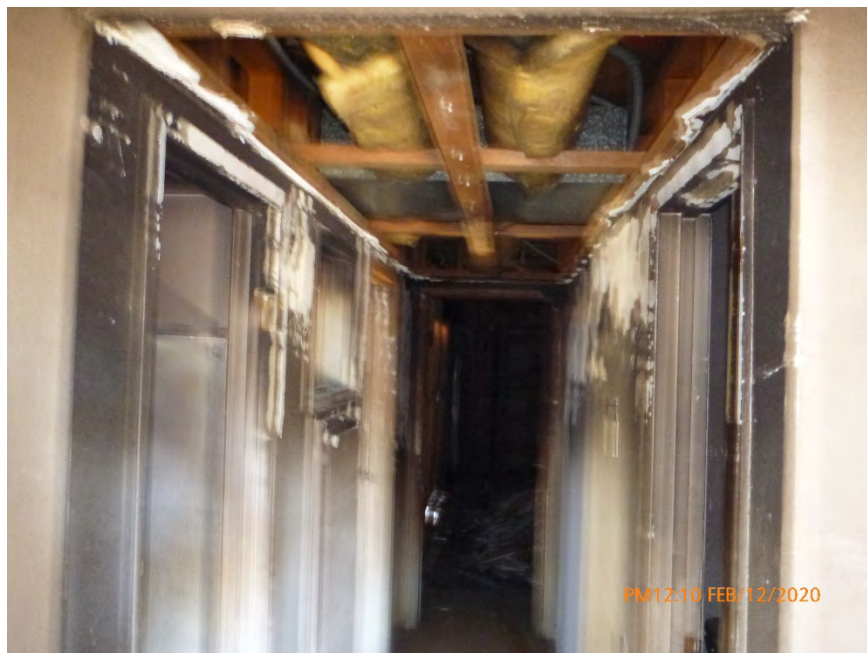
Photograph 21: February 12, 2020, at approximately 12:10 PM - View of a hallway in Unit 3 where acoustic ceiling texture ( ACT ) had been removed from the ceiling. The ACT on the ceiling was a Regulated Asbestos-Containing Material.
